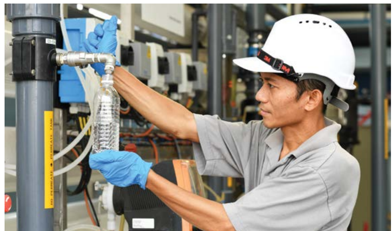
Nestlé employee monitoring water quality using the Direct Potable Reuse System (DPRS)
