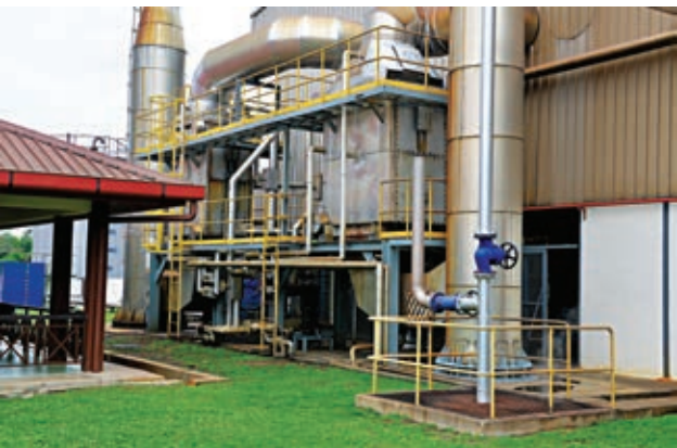
The Economiser is used to recover potential energy emitted from the boilers at our factories.
