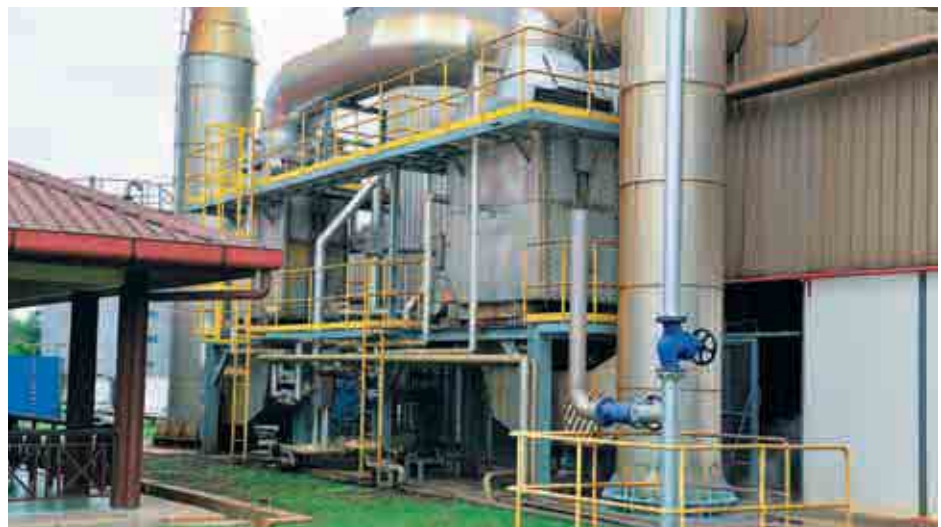
The Economiser is used to recover potential energy emitted from the boilers at our factories.
